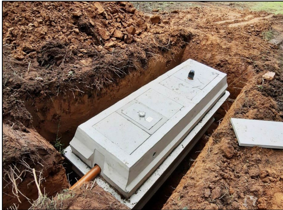
Plate 4-12: Typical wastewater holding tank used on wind farms
