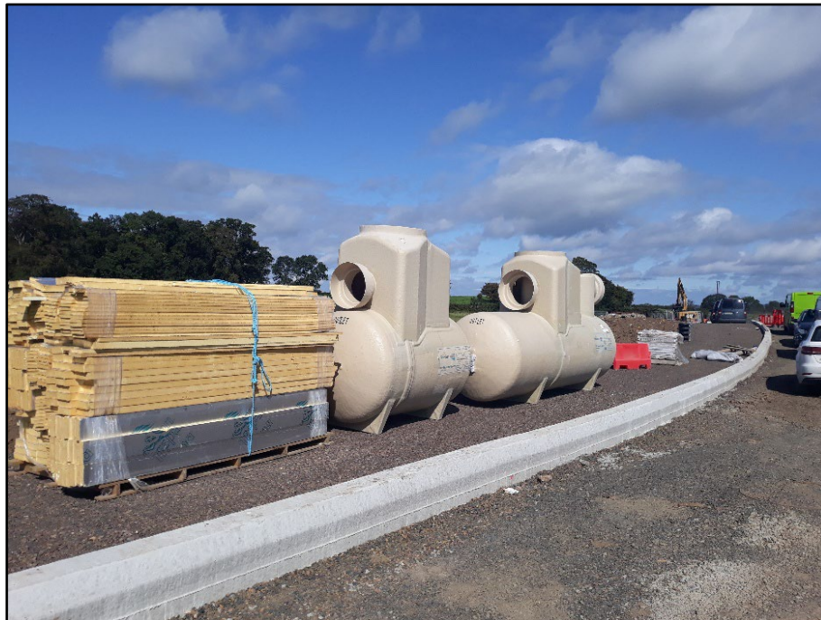
Plate 4-8: Typical proprietary treatment device used on wind farm substation compounds
