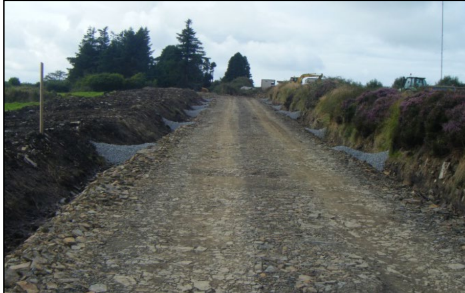
Plate 4-14: Typical conveyance swale feature used within wind farms
