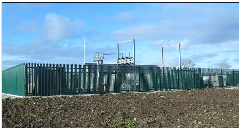
Plate 4-5: Example of a typical substation building and compound
